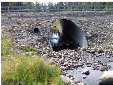
Figure 15. Round culvert. Photo: Erik Degerman
