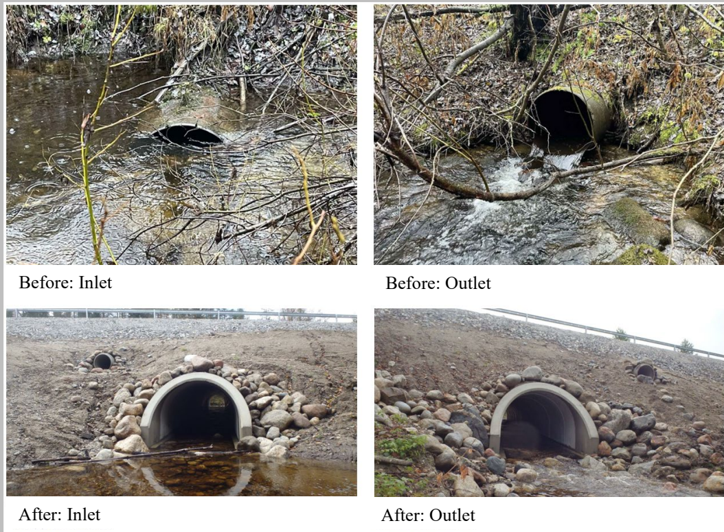
Figure 16. Example of before and after a remediated road culvert by beneficiary STA. The smaller culvert in the after pictures is an otter passage.
